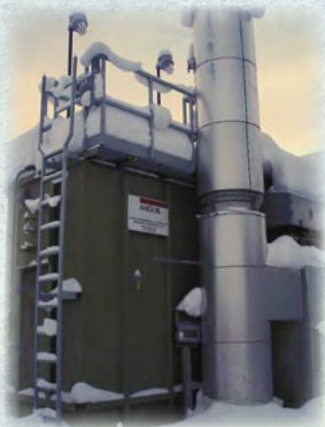
This Anguil incinerator burns vapors collected during the ballast water treatment process. Two such units have been installed at the Ballast Water Treatment Facility. Photo by Tom Kuckertz.
