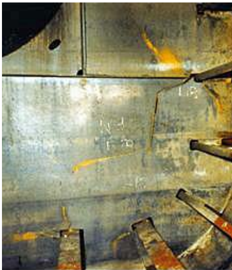
Figure 4.2 Example of fatigue crack (from single hull tanker)
