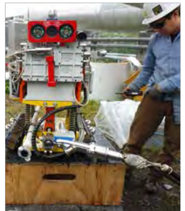
Alyeska staff implement new technology that can inspect areas of pipe that were previously impossible to inspect. Photos courtesy of Alyeska.
