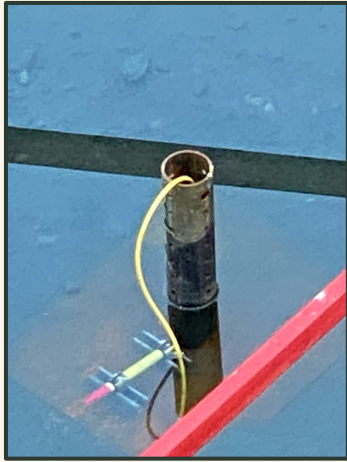
Standpipe with piezometer and RBR Pressure Transducer
