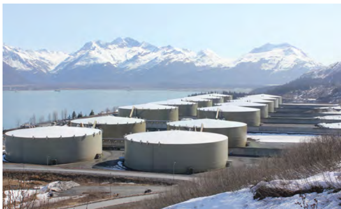
A secondary containment system surrounds the oil storage tanks to hold oil in case of a spill.
