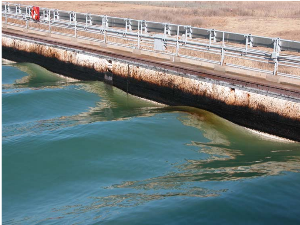
Figure 2: Oil stains on tank wall
