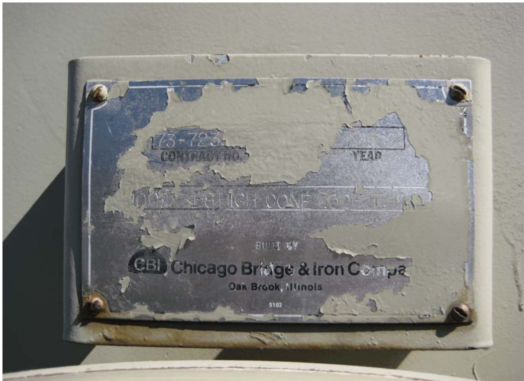
figure 2 - 58-TK-55 tank nameplate. The contract number (73-7235) and build year (1976) are legible.
