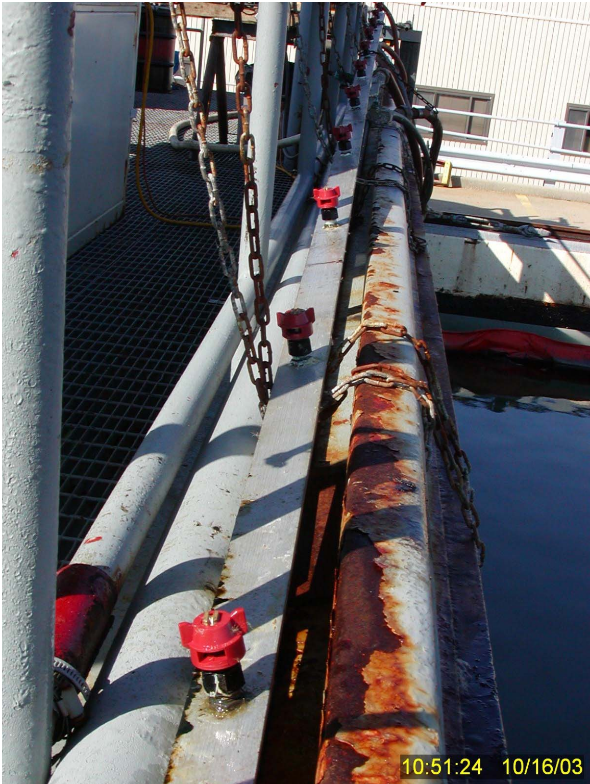
Figure 249 UniJet Model No. 8001 flat spray nozzles mounted on the dispersant spray bar while it was pulled up to the movable bridge rail for adjustment in preparation for Test No. 20.
