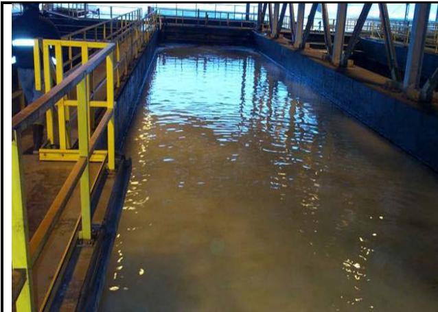
Figure 9: BWTF Dissolved Air Floatation (DAF) cells
