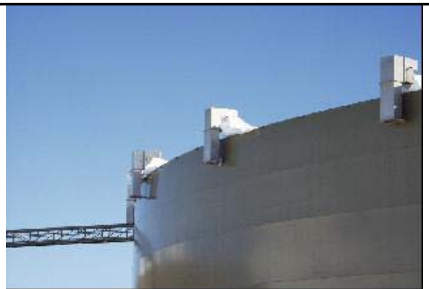
Figure 4: closer view of oil storage tank vents
