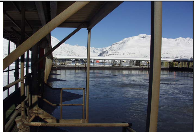
Figure 10: BWTF Biological Treatment Tank (BTT)
